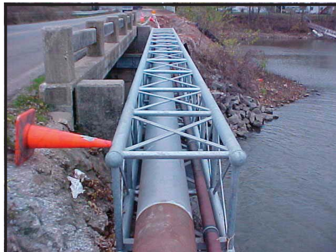
Delaware CO RWD #10- A water line going across a bridge crossing on Grand Lake.
